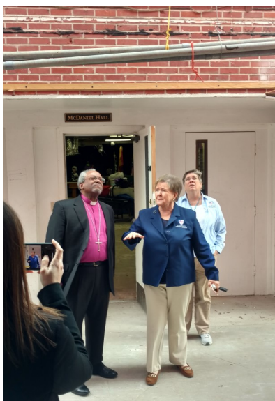
Bishop Curry looks at damage to the north end of the Bill Lloyd Building with Mrs. Hughes & HNES Business Manager Kathy Mills.
