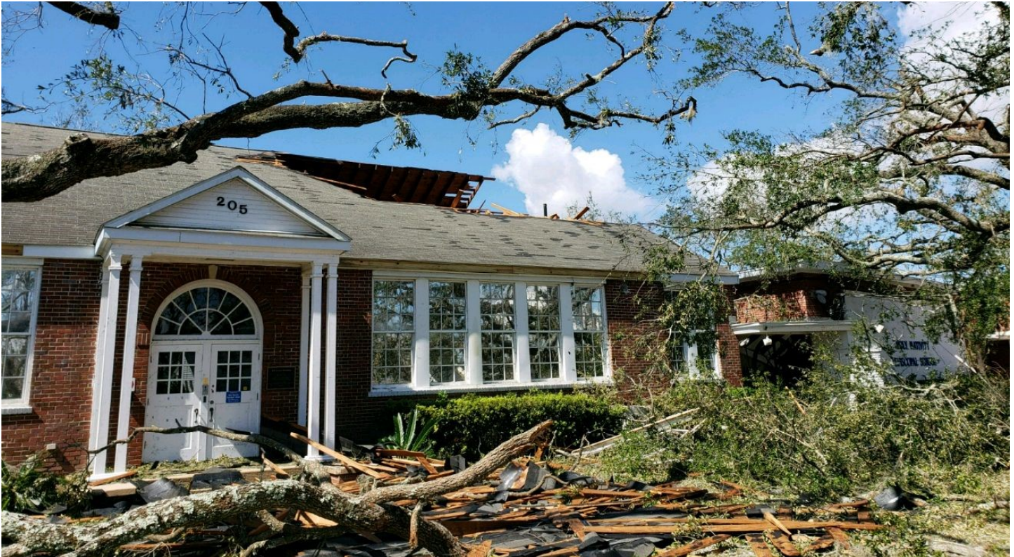
The heavily damaged portion of the 1937 Cove Schoolhouse at 205 Hamilton Avenue is shown in this October 11, 2018 photo
